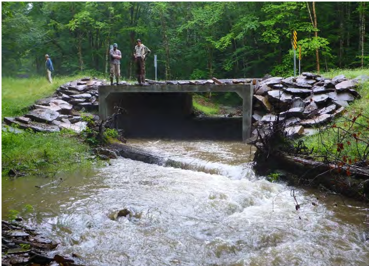
Road crossings that can withstand flood events (USFS, Monongahela NF)
